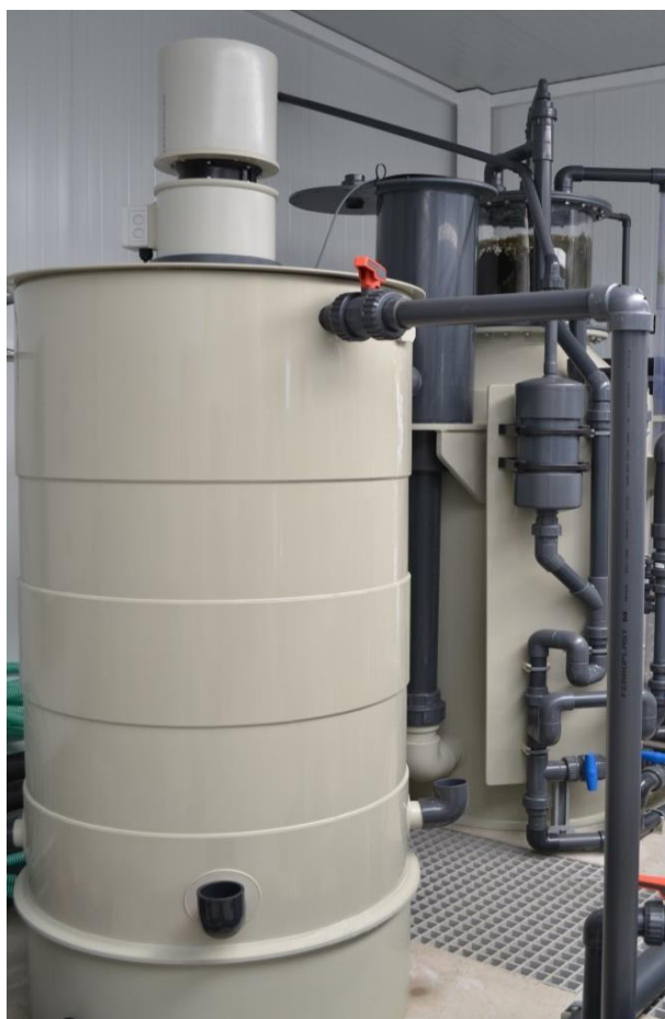
Fig. 9 – Trickling filter used at RiaSearch for ammonia removal and carbon dioxide degassing. Photography courtesy of Adriana Laranjeira, RiaSearch.
