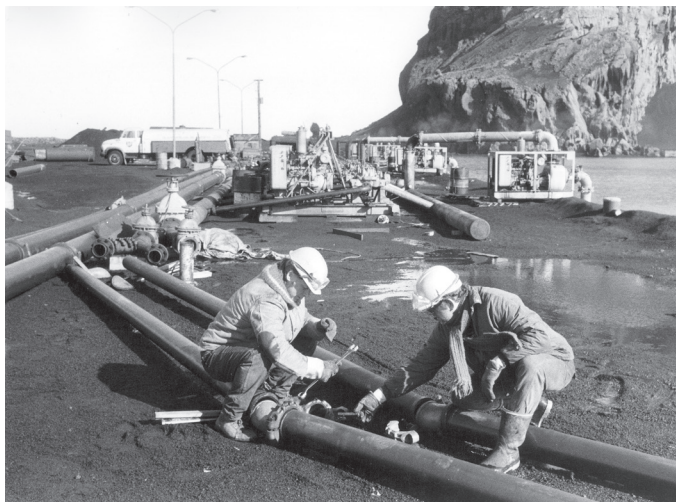
Fig. 22. Pumps and pipes on the harborside. Photo by Sigurgeir Jónsson.
