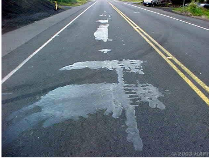
Figure 1-4. An example of bleeding on flexible pavements (Pavement Interactive website)
