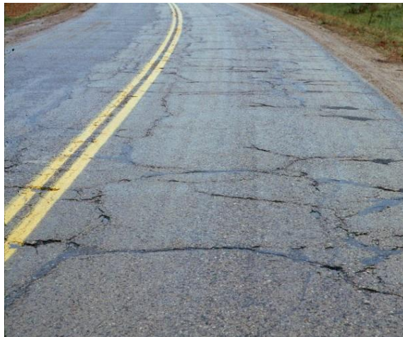
Figure 1-2. An example of block cracking on flexible pavements (Pavement Interactive website)
