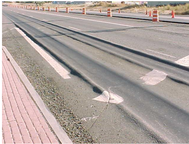
Figure 1-5. An example of rutting on flexible pavements (Pavement Interactive website)
