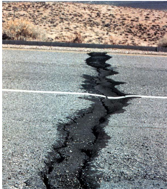
Figure 1-1. An example of very severe low temperature cracking on flexible pavements (Pavement Interactive website)
