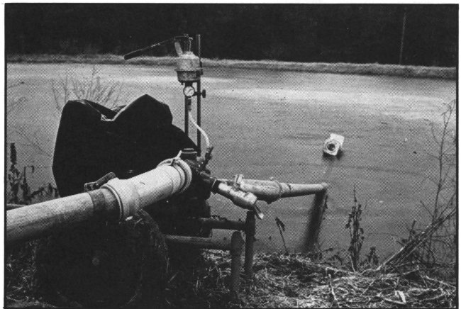
Figure 11. A pump intake floated 1-2 feet, below the surface will be least likely to plug.
