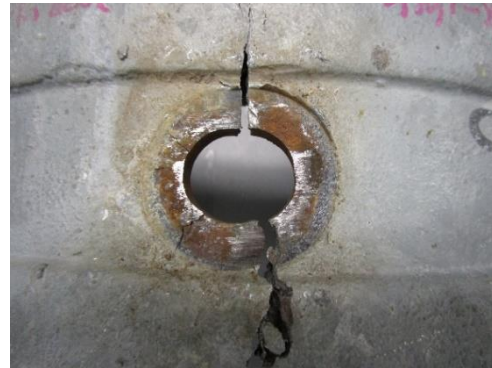
(b) Cracked 10-in. Coupler
