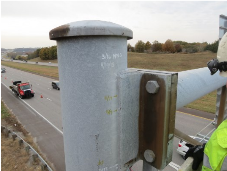
Figure 2 Typical crack monitoring at the box connection of a two-chord COSS
