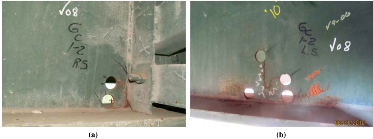
Figure 9: Cracking at the instrumentation location on the (a) stiffener side (b) non-stiffener side.
