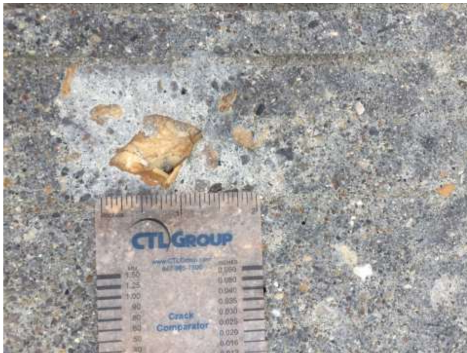
Figure 5.9: Surface damage on IN-IC-HPC-3
