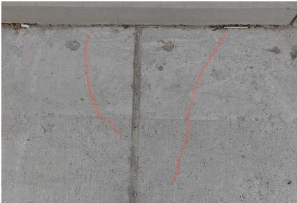
Figure 4.11: IC-LC-HPC-1 typical crack pattern
