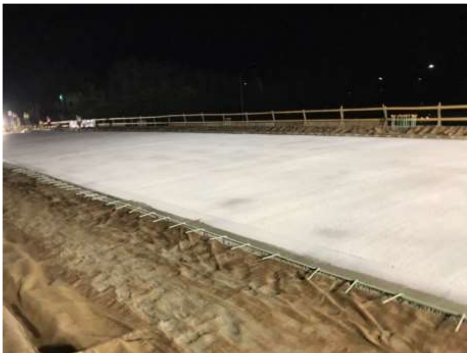
Figure 4.10: Finished IC-LC-HPC-4 deck showing spots of uneven curing compound application
