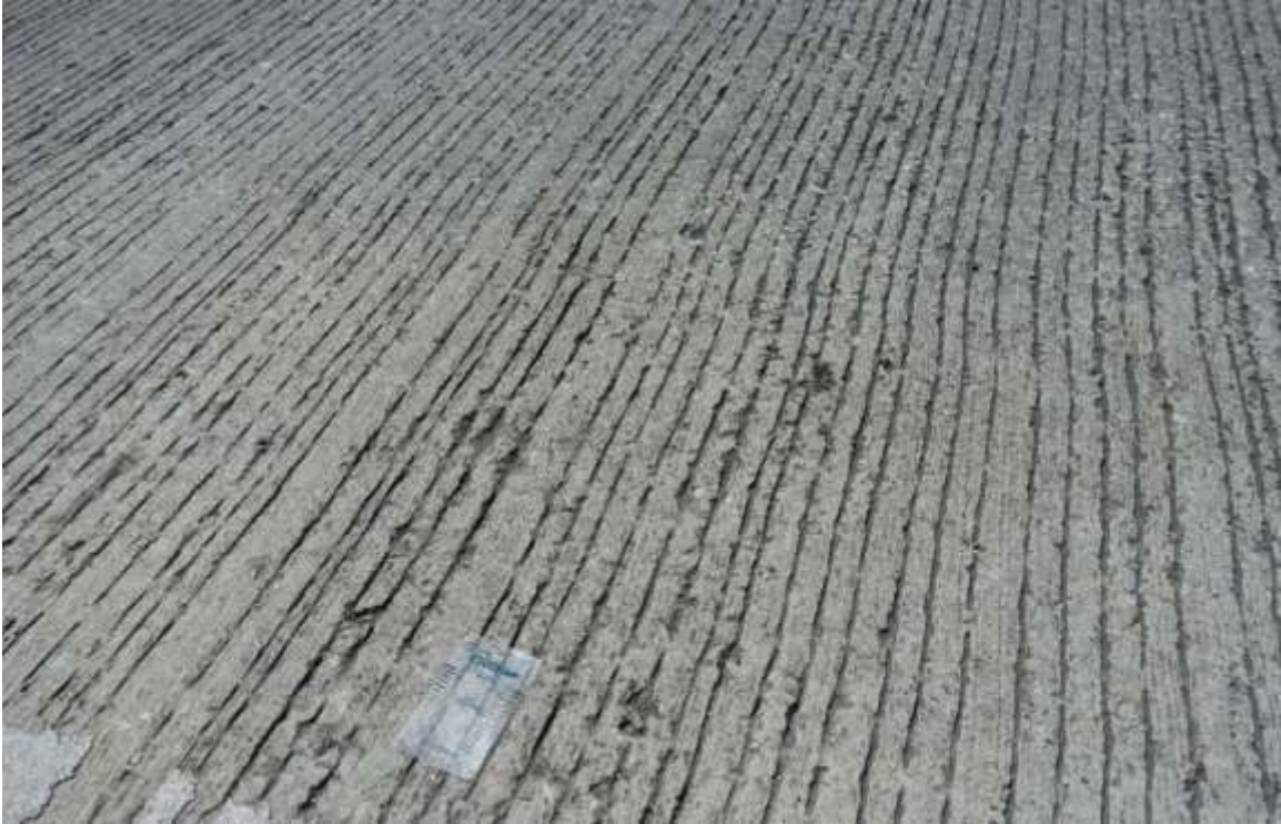
(a) Freeze-thaw damage
