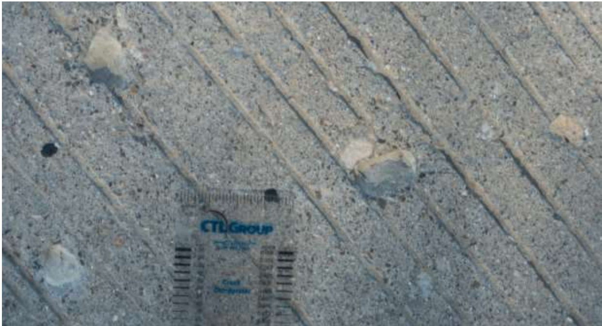
(b) Aggregate popouts (the crack width comparator has a width of approximately 2 in. [50 mm])
