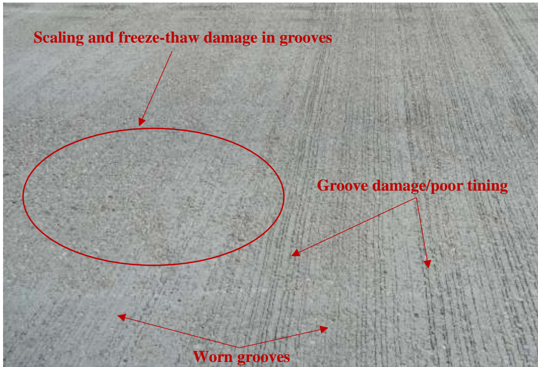
Figure 5.11: Freeze-thaw damage (aggregate popouts) and uneven tining on IN-IC-HPC-4 apparent in 2016
