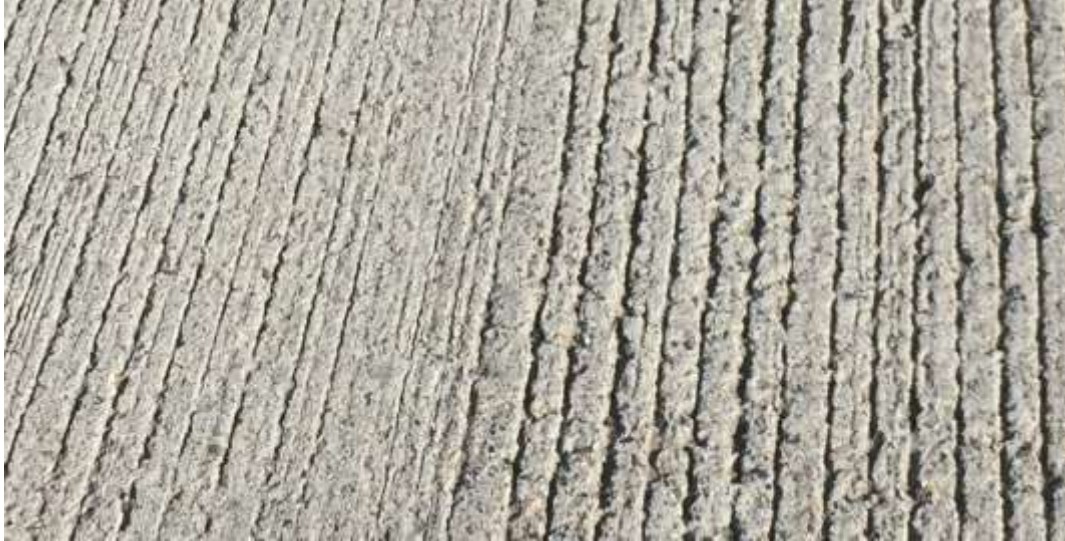
Figure 4.18: Poorly tined area on IC-LC-HPC-4
