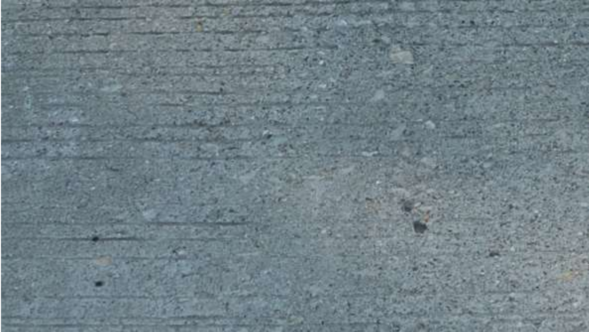
(a) Scaling near the north end of IN-IC-HPC-1
