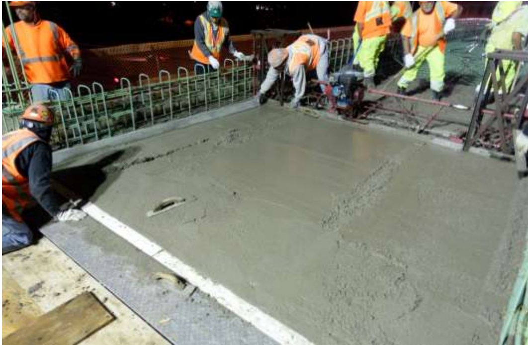
(a) Surface imperfections at the north end of the deck after first screed pass
