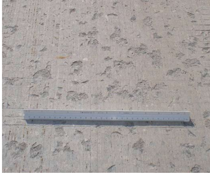
Figure 1.3: Scaling of concrete (Lindquist et al. 2008)
