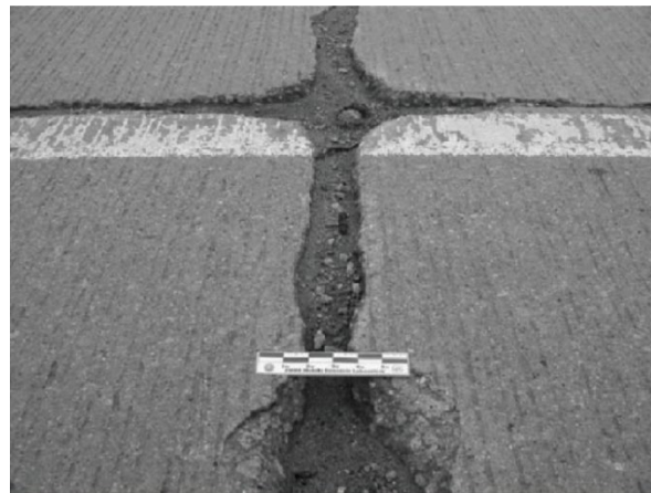
Figure 1.1: Damage at joint (Jones et al. 2013)
