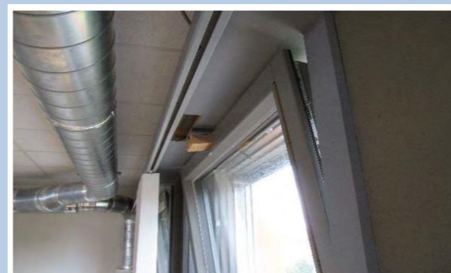
Fig. 4. Detail of motorized window for Night Ventilation in Case study 1 Building
