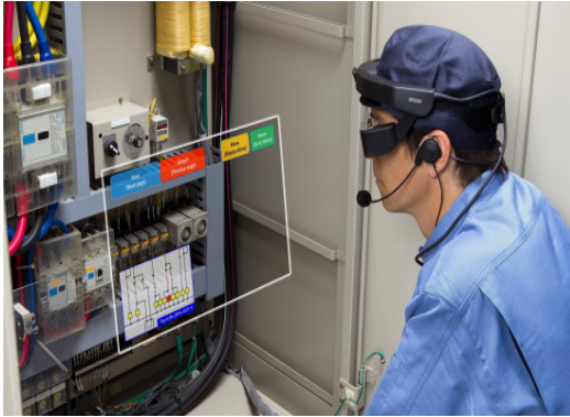
Figure 14. “With the number of diverse devices residing in a typical substation these days – some new and some very old – it is nearly impossible to have at hand all of the relevant maintenance and repair data in the form of hard-copy manuals and papers to get the job done,”(Judson, 2017). (Image: https://blogs.cisco.com/energy/augmented-reality-a-new-reality-for-utilities )
