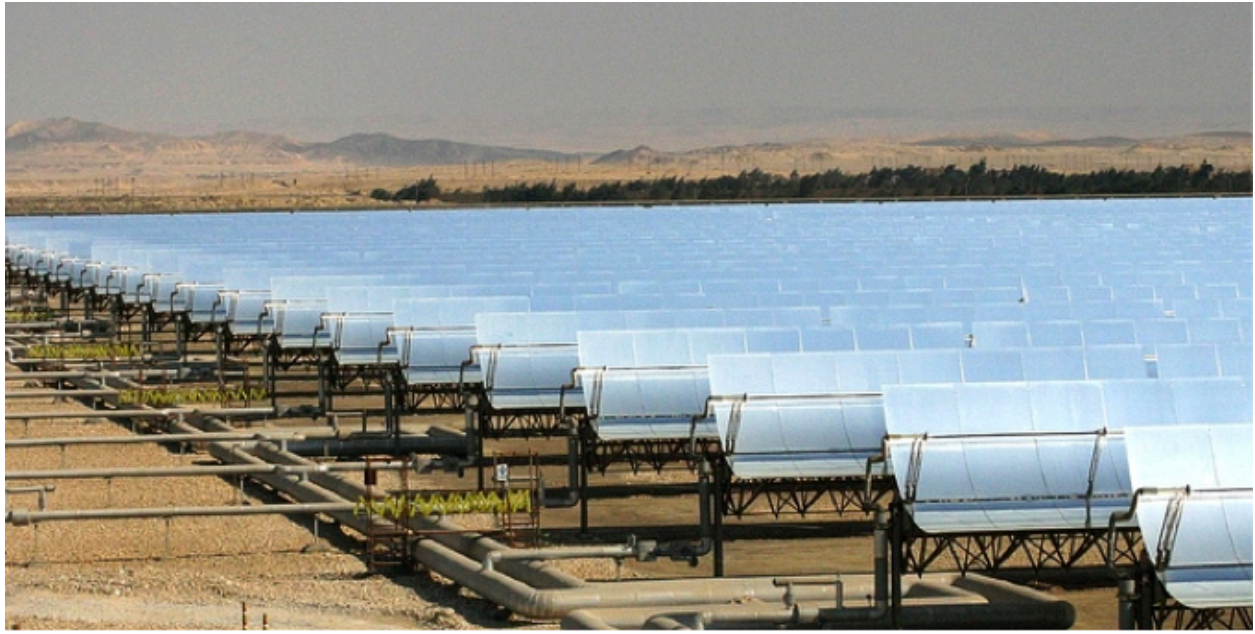
Figure 3: Kuraymat parabolic trough solar power plant
