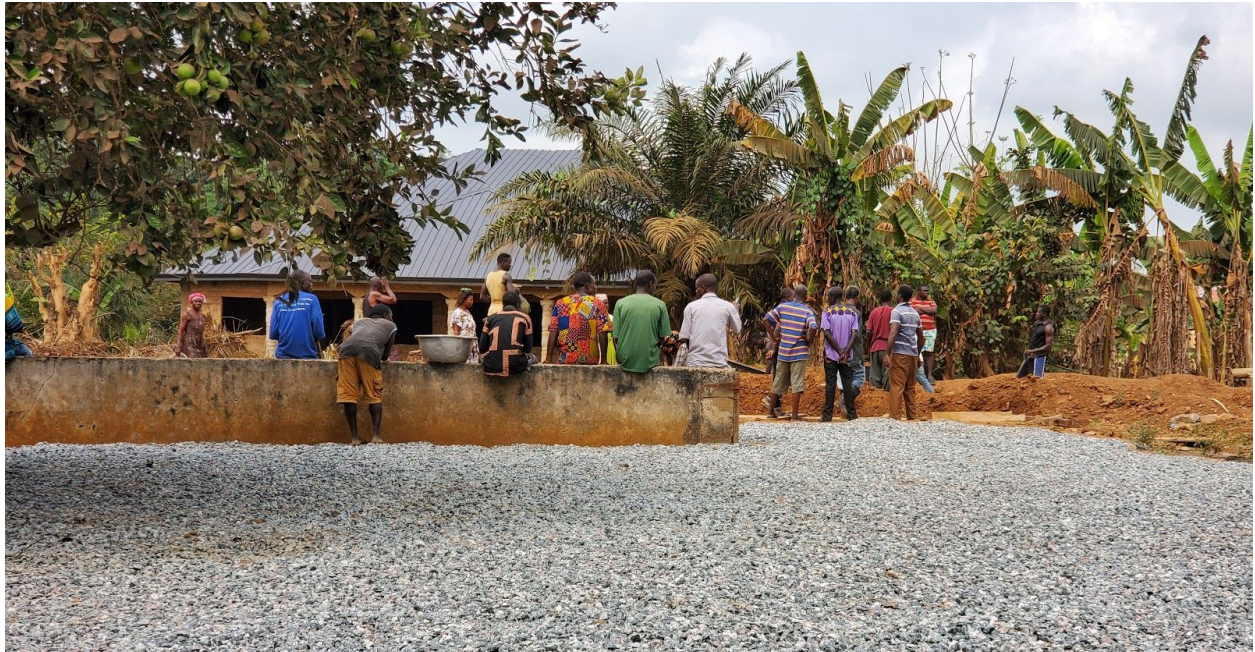
Figure 2: Community members working together on the road to the Dwenase Health Center.
