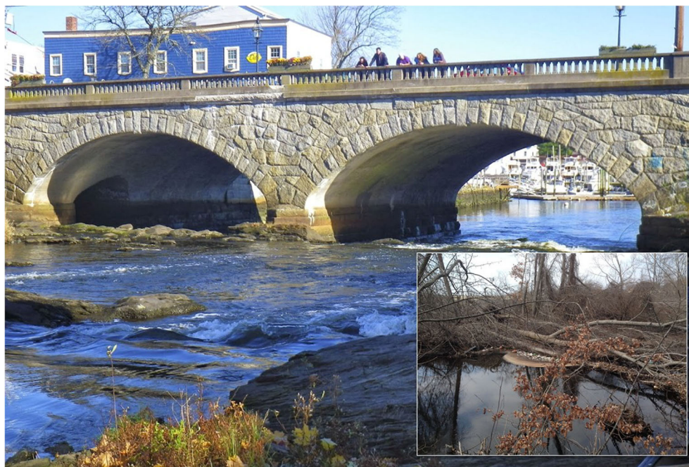
FIGURE 5 A snapshot of the Pawtuxet Village Bridge and some wood debris upstream of this bridge in the river channel that might be mobilized during a flooding event
