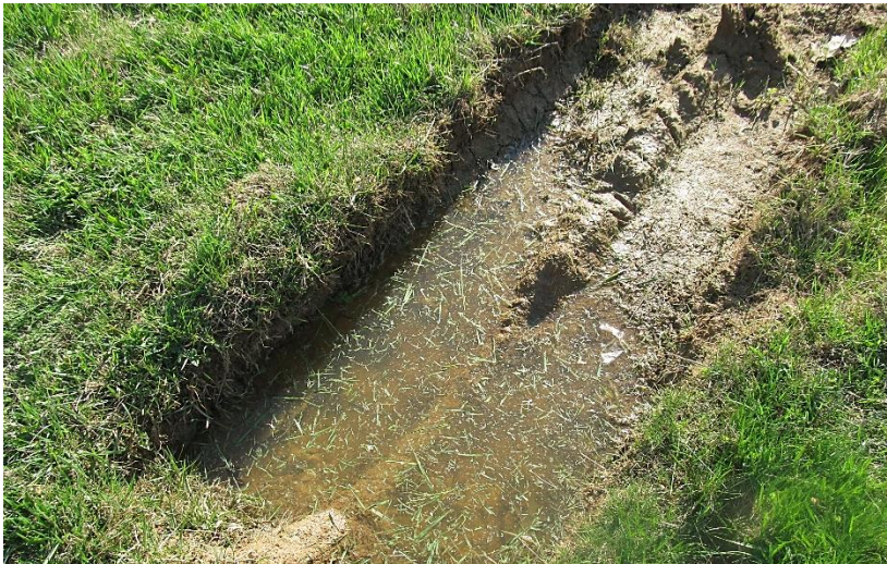
Figure 31. Muddy areas around the community garden that is the result of insufficient stormwater management strategies
