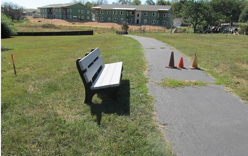
Figure 30. Damage that runoff has caused along the walking paths
