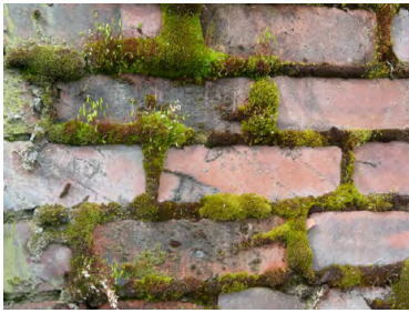
Figure 1a. Biogrowth1: Approximately seven bricks with significant growth of moss and discolored surfaces.
