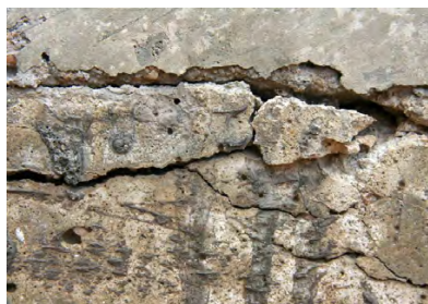
Figure 1k. Concrete1: Close-up of concrete wall with deep, irregular cracks and surface soiling.
