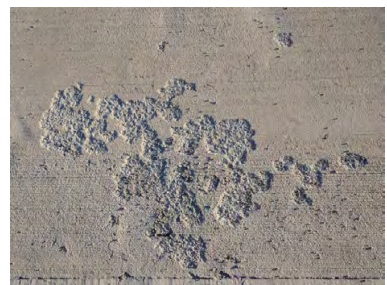
Figure 1l. Concrete2: Close-up of concrete wall with surface erosion.
