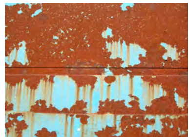
Figure 1u. Ferrous2: Close-up of steel sheet with significant surface rust and eroded blue paint.
