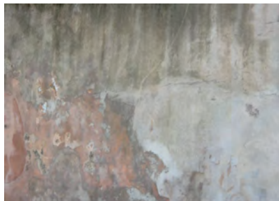
Figure 1w. Stucco1: Smooth stucco wall with significant soiling and irregular surface discoloration.
