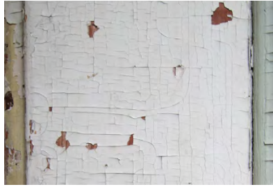
Figure 1z. Paint1: Close-up of painted piece of wood with alligator cracking.
