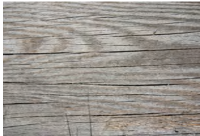
Figure 1ac. Wood1: Close-up of unpainted wood floor with UV-damaged (gray) surface and cracks.
