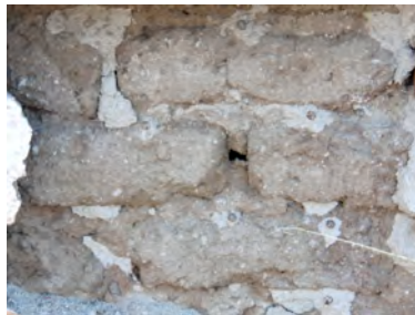
Figure 1q. ExposedEarth2: Approximately four large adobe blocks with some surface erosion.
