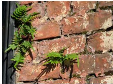
Figure 1b. Biogrowth2: Approximately seven bricks with decayed surfaces and mortar with small ferns growing in mortar joints.
