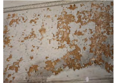
Figure 1aa. Paint2: Close-up of painted wall with significant paint loss due to alligator cracking.
