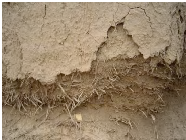
Figure 1p. ExposedEarth1: Close-up of adobe (earth) wall with lower section significantly eroded, exposing interior straw reinforcement.
