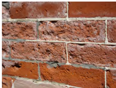
Figure 1e. Brick1: Approximately seven bricks with decayed (rough) surfaces and damaged mortar.
