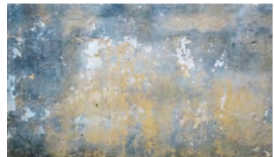
Figure 1x. Stucco2: Slightly irregular stucco wall with significant soiling and surface erosion.
