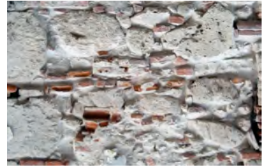
Figure 1o. ExposedRubble2: Close-up of interior of brick and stone rubble wall construction (stucco surface has been removed) with white lime mortar.
