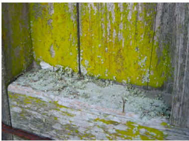
Figure 1d. Biogrowth4: Close-up of wood fence with significant lichen growth.
