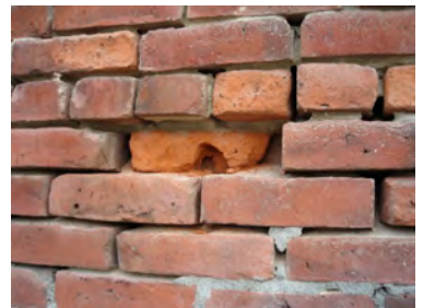
Figure 1f. Brick2: Approximately twelve bricks with eroded mortar and one damaged brick.
