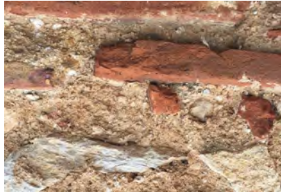
Figure 1n. ExposedRubble2: Close-up of interior brick and stone rubble wall construction (surface stucco has been removed) with beige lime/earth mortar containing lime blebs.
