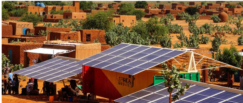
Figure 28: Solar container from Africa GreenTec at Amaloul, Nigeria
