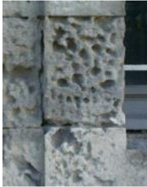
Figure 13- damages due to biological mechanisms
