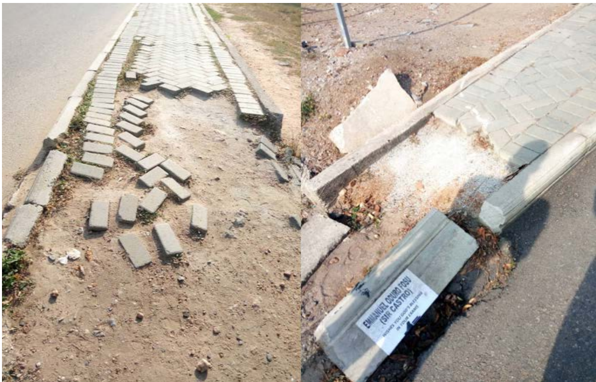
Figure 5.2: Walkways with broken and dislodged bricks in PUB
