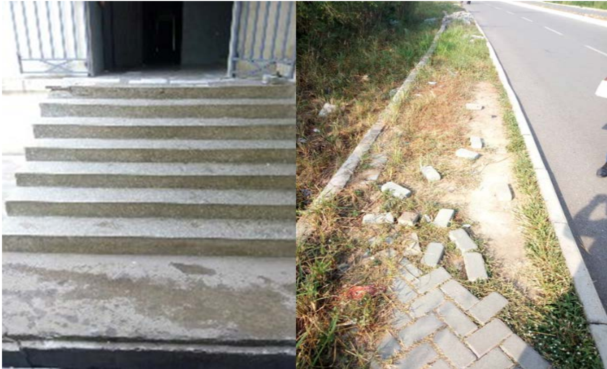
Figure 5.1: Stairs leading to a bathroom in a university hall of residence in PUB (left) A walkway with hazards in PUB (right)
