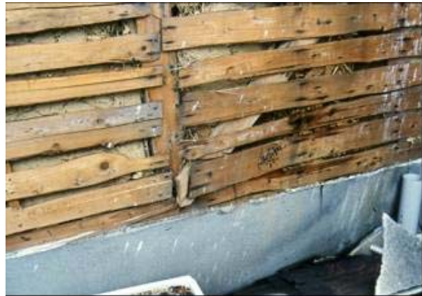
Fig.5 Poor connection between brace and sill or column observed in the 1955 Great Hyogoken-nanbu earthquake.
