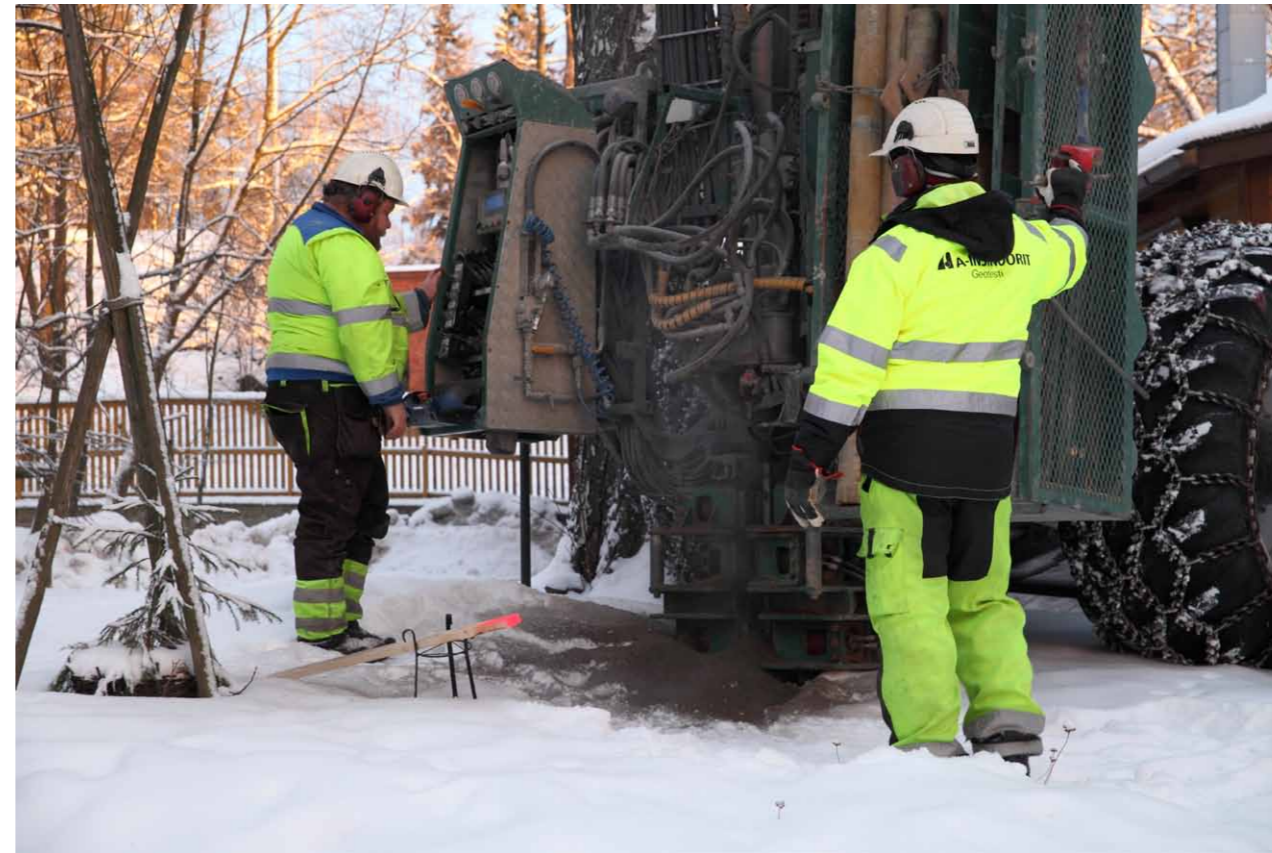
Picture 4.1. Drilling to determine the rock surface in January 2013. Source: Rantatunneli Alliance
