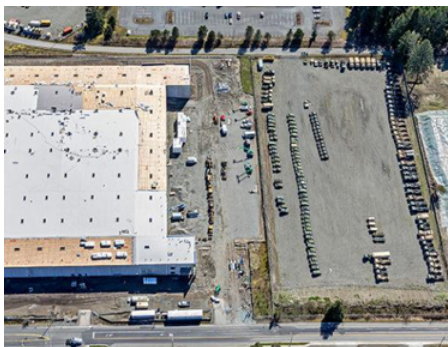
Bridgepoint I-5 in the East Columbia Corridor off of Marine Drive by Bridge Development http://www.sierraind.com/projects/bridge-point-i-5/
