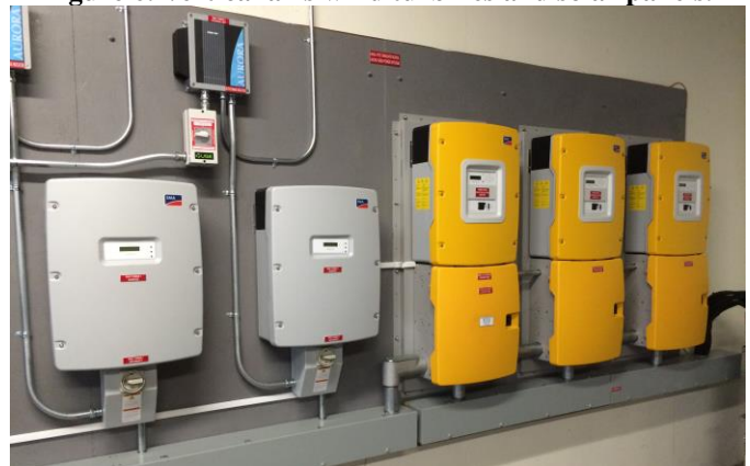
Figure 7. Installed 3 phase 208V microgrid.
