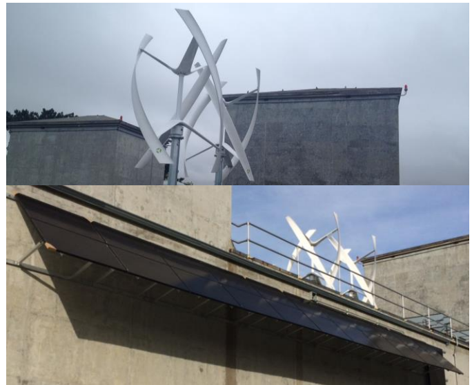
Figure 6. Vertical axis wind turbines and solar panels.
