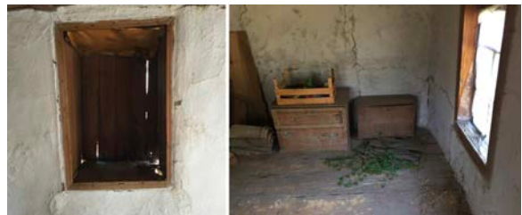
Figure 28: Left - View of a niche for ritual washing (abdesthanu) from divanhana; Right - Small room (oriented to the "house" ("kuća")). It also served as a pantry ("huderu")
