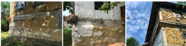
Figure 18: Details of the structural assembly of the house; Left and center - Basement wall of semi-finished stone; Right - Bondruk system with adobe fill (ground floor and first floor)
