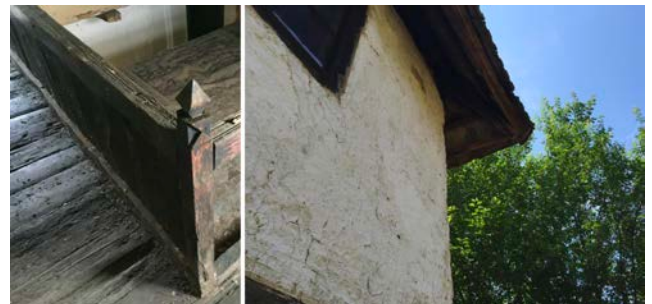
Figure 17: Left - Detail of fence on gallery; Right - Finishing of exterior wall surfaces: white painted clay mortar with straw and chaff
