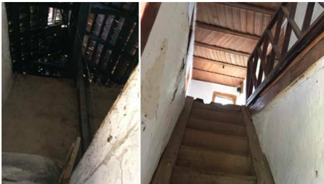
Figure 14: Left - View from the “house” (“kuća”) space towards the garret and roof; Right - View from entrance windshield to staircase to floor and divanhana
