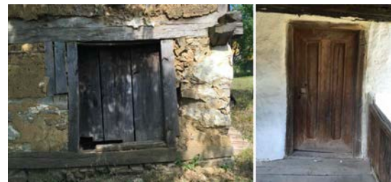
Figure 22: Left - Door on the basement wall; Right - Entrance door to the house (from the porch on the southeast side of the house)
