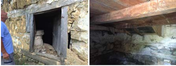
Figure 6. Left - entrance to the storeroom ("magaza"); Right - basement area. Below the ceiling, in the corner, you can see a special structure with a thick layer of slag that has been made under the brick oven in the room. It was a fire protection of the wooden elements of the floor basement-ground floor structures
