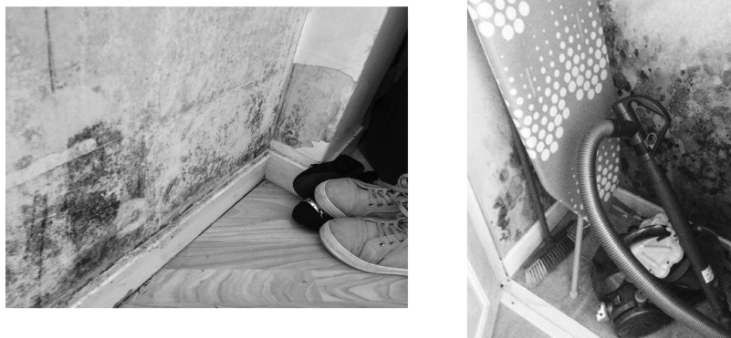
Figure 6 Left: mould growth and dampness. Right: dampness in a child's bedroom.
