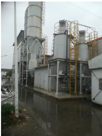
Air filtering system, right outside the smaller buildings/rooms.
