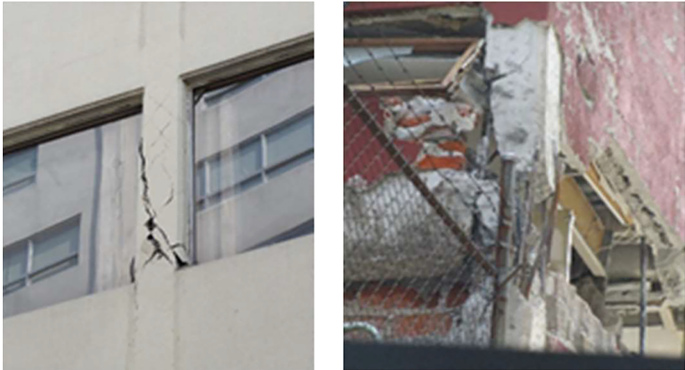
Figure 3. Examples of structural damage in buildings surveyed by CICM and SMIE (2017).
