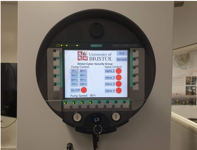
(b) A Siemens Mobile Panel 277 IWLAN V2, mounted on cabinet
