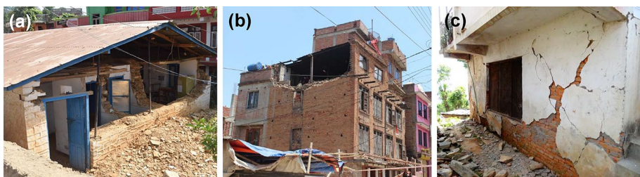
Fig. 3 a URM-SM OOP damage (credit: Suraj Shrestha, EERI photo archive), b URM-BM OOP damage at higher story (credit: Bipin Shrestha, EERI photo archive), c URM-BC IP damage (credit: Bret Lizundia, EERI photo archive) (EERI 2019)
