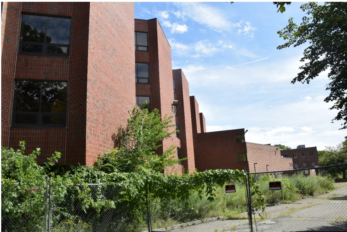
Above: Back of the hospital, adjacent to the wooded Medford portion, which might have been an access point for ambulatory vehicles.
