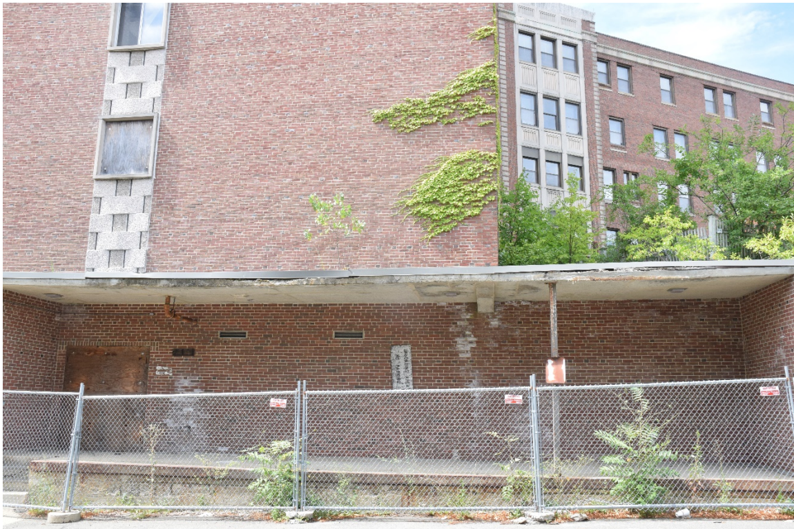
Above: Former loading dock at the side of the hospital, from Hospital Road.
