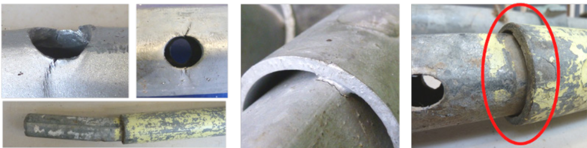
Figure 3.51: Modes of failure. Left: Plastic deformations around spigot holes, Centre: cracks in welds, Right: slippage of the spigot.
