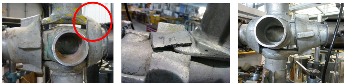
Figure 3.44: Modes of failure. Left, Bottom cup, Centre, top cup, Right, slippage of the ledger.
