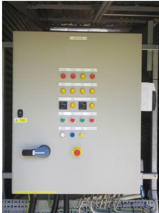
Figure 4-7 – Pump Room Control Box
