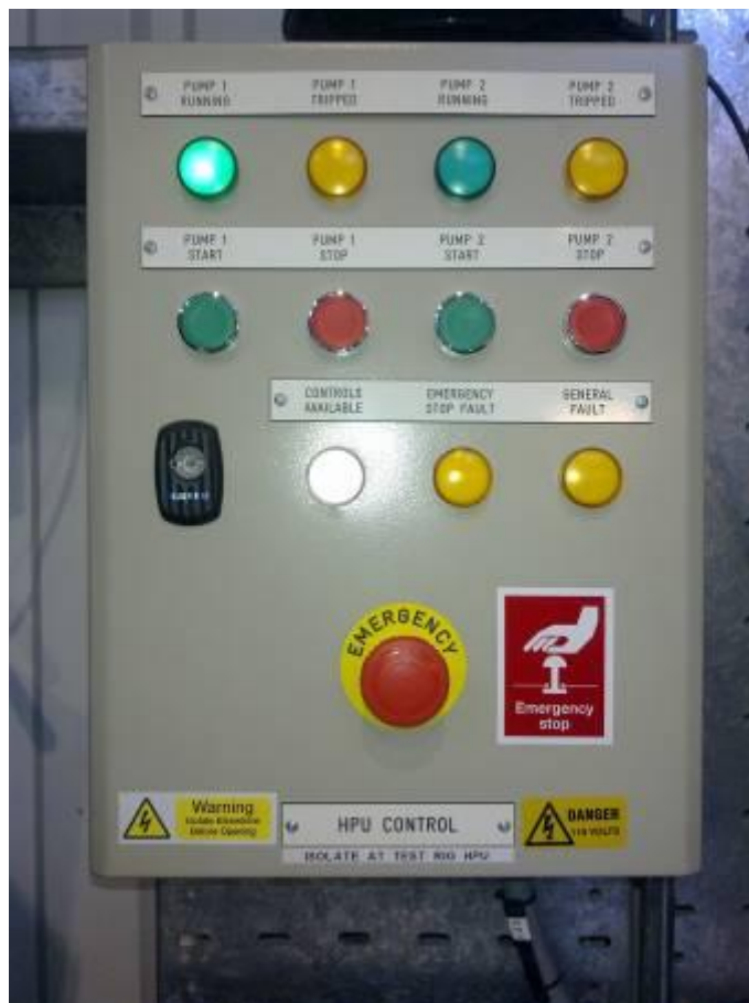
Figure 4-8– Four-post Rig Pump Control Box
