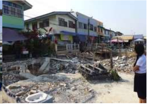
Development of new open space in the process in Saphan Mai (case 2)
