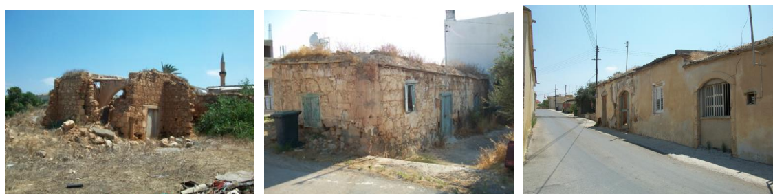
Figure 7.9: Examples of demolished and vacant Greek Cypriot houses, Akdeniz/Agia Eirini.
