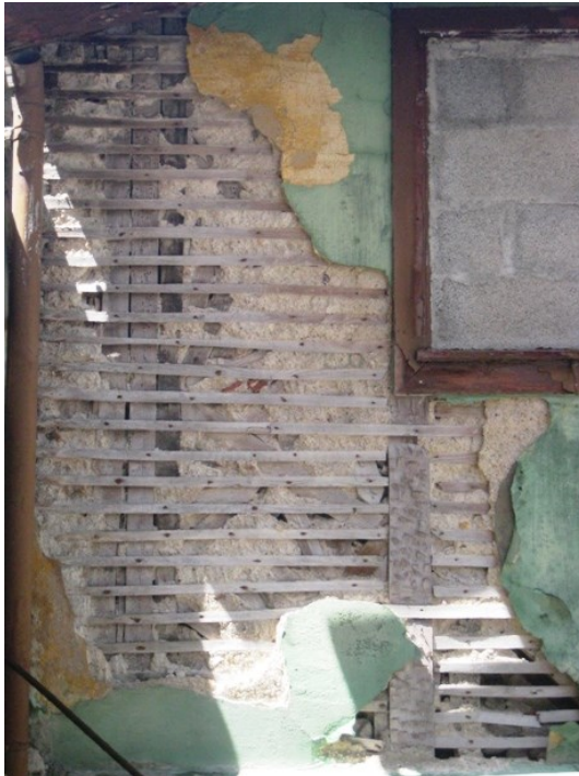
Figure 29 – Exterior timber stud wall framing with lath and plaster in a ruined building
