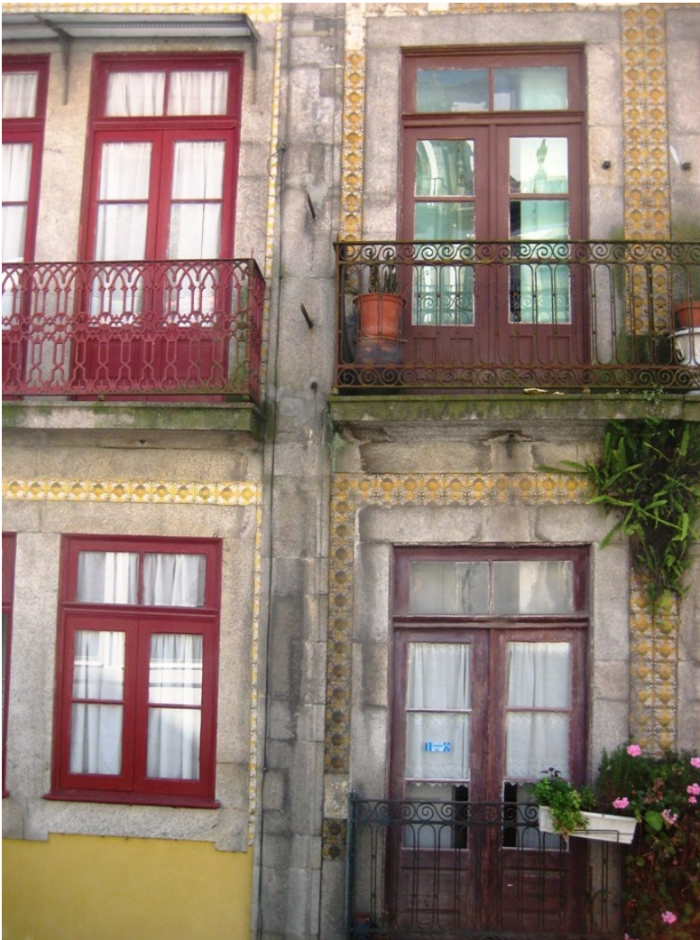
Figure 67 – Original balcony door with special glass in a traditional building in Oporto
