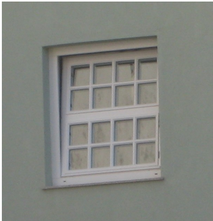
Figure 66 - Wood frame imitating the traditional sash design in a traditional building in Oporto
