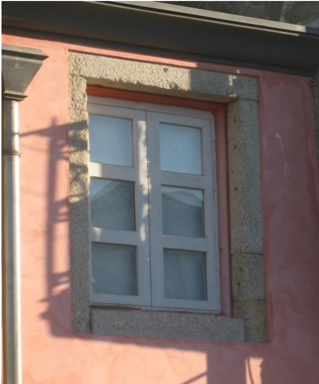
Figure 62 – Historic centre building in Oporto where plaster is above the granite jambs
