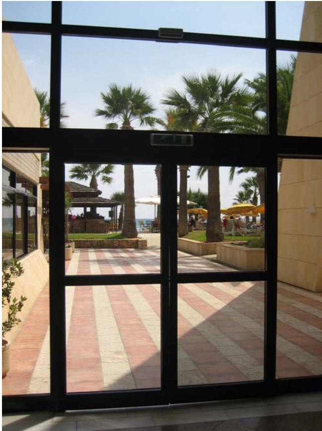
Figure 7.21 Double doors of the case study hotel model showing poor air-tightness
