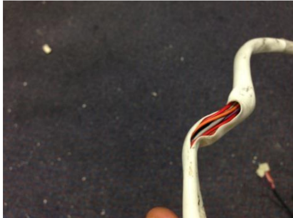
Figure 5.26 - Cracked outer cable on a loom
