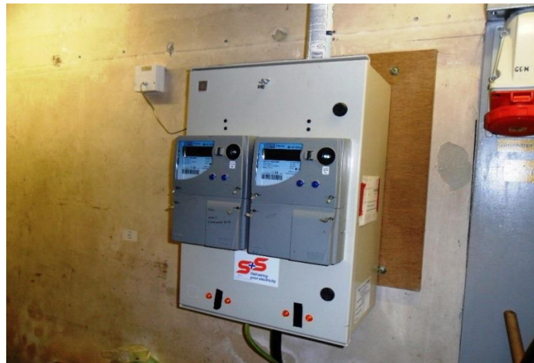
Figure 59 - Primary electric and verifier meters
