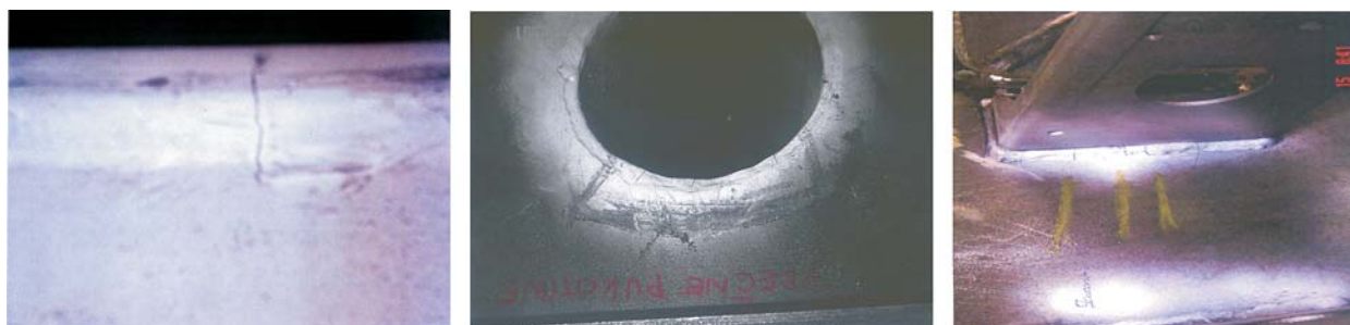
Figure 2 Cracks on welded structures made of S 960 QL steel Slika 2. Pukotine na zavarenim konstrukcijama od čelika S 960 QL
