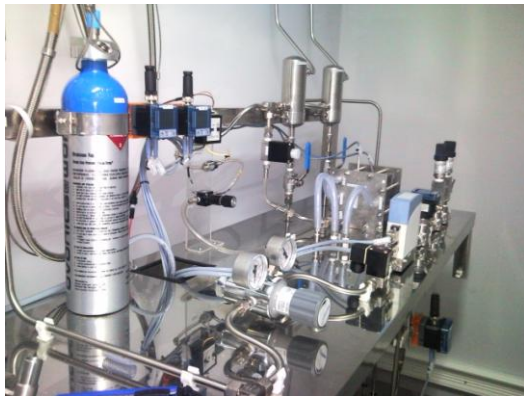
Fig. 10: Part of the hydrogen unit placement.
