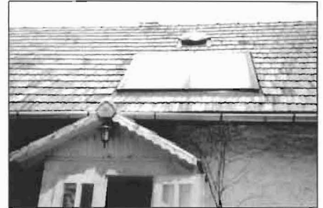
Image 13: Solar panels on the roof for heating water and providing electricity
