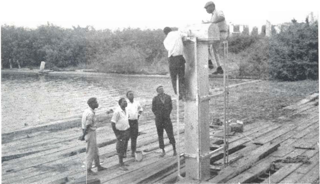
Installation of level recorder at Butiaba on Lake Albert
