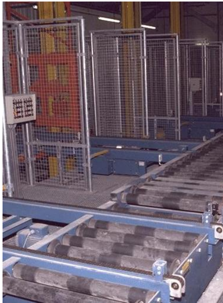
Fig. 1 Pallet elevators at the distribution center of Herlitz with a single waiting slot in front of each
