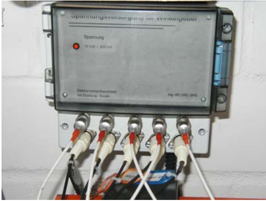
Figure 4.13: Constant voltage supply unit
