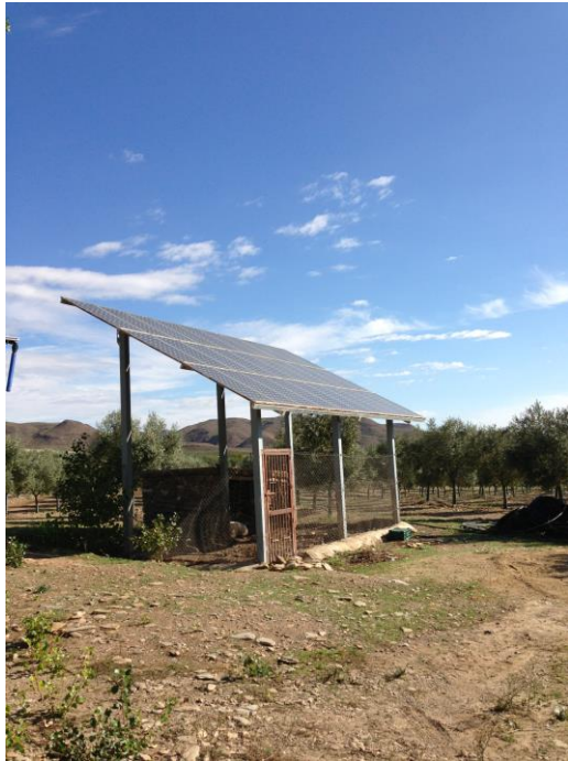
Plate A. Solar Photovoltaic Panels
