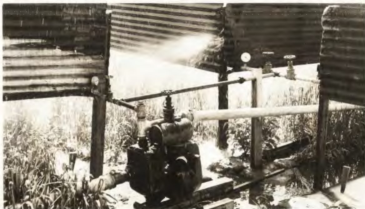
Figure 5. Pump, valves and pressure guages. A valve and pressure guage was provided for the regulation of water application to each plot.
