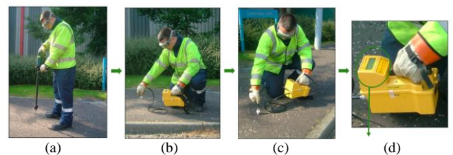
Figure 3. Process for Pinpointing Cable Faults Using Cable Sniffer Method: (a) Make a hole in the surface (b) Insert probe (c) Draw gas from below the surface (d) Sniffer analysis of gas
