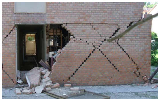
Figure 17. Failure mode of a building made of bricks and cement mortar (San Possidonio, Italy).
