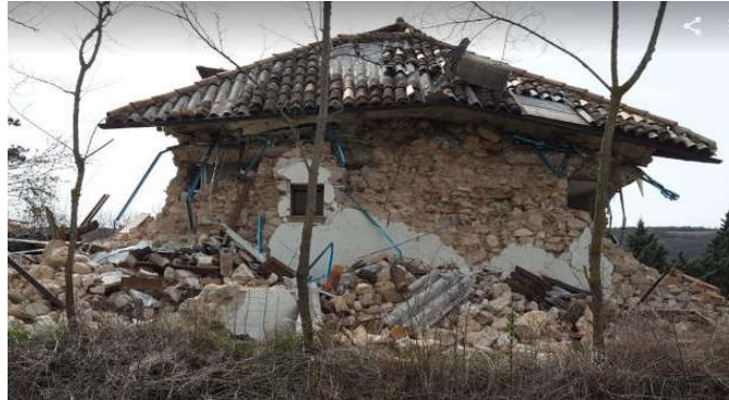
Figure 8. A collapsed building in Campi Basso, Norcia, Italy: The masonry (combination No. 1 of Table 4) of this building disaggregated during the earthquake.
