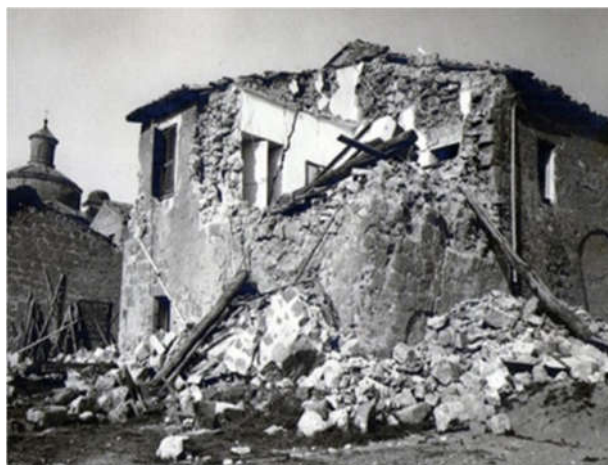
Figure 12. Tuff stone building in Tuscany, Italy, after the 1971 earthquake: the masonry typology can be classified in combination No. 1 of Table 7: irregular stones, non-horizontal bed joints, unconnected wall leaves, and very weak mortar. The failure mode is by disaggregation.
