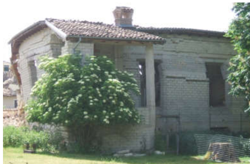
Figure 16. A building made of concrete block and irregular stones in Onna, Italy.
