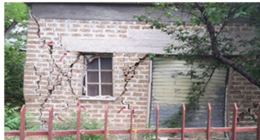
Figure 13. Tuff block masonry of a building in Norcia, Italy: the quality of the mortar is good (combination No. 6, Table 8). The 2016 earthquake caused the shown failure mode: it can be noted that cracks diffusively opened in the tuff blocks, while this is very rare if the mortar quality is weak. Masonry disaggregation usually does not occur for this masonry typology.
