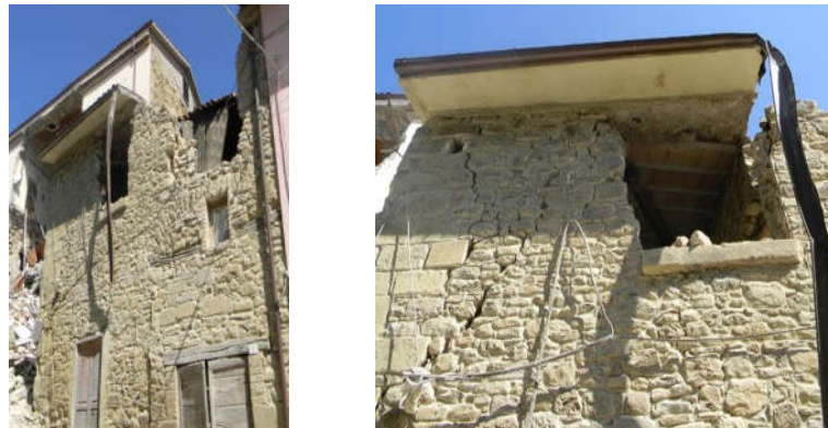
Figure 10. A building in Accumoli, near Rieti, in Italy: a large number of large cut stones was used here. This highly increased the level of connection between the wall leaves (combination No. 7, Table 5: cut stone masonry, medium-quality mortar, and effective connection between wall's leaves). For the upper part of this building, the quality of the masonry is lower and the wall leaves seem unconnected (combination No. 5, Table 5: cut stone masonry, medium-quality mortar, and non-effective connection between wall's leaves). The masonry of the upper part of this building disaggregated during the 2016 Central Italy earthquake.
