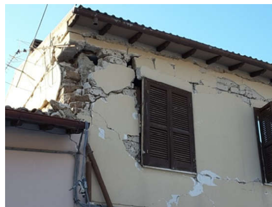
Figure 14. A tuff masonry building in San Pellegrino (Norcia, Italy): the masonry was made of squared tuff blocks and a very weak mortar (combination No. 2, Table 8). Cracking mainly occurred in the bed joints. The 2016 Central Italy earthquake caused a failure mode by horizontal sliding of the upper part of the building, likely activated by significant vertical component of the seismic action. The phenomenon of masonry disaggregation can be noted at the corner.
