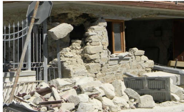
Figure 11. Pescara del Tronto, near Ascoli Piceno, in Italy. This is an example of cut-stone masonry, very weak mortar, unconnected wall's leaves (Combination No.2, Table 6). The building failed due to masonry disaggregation.
