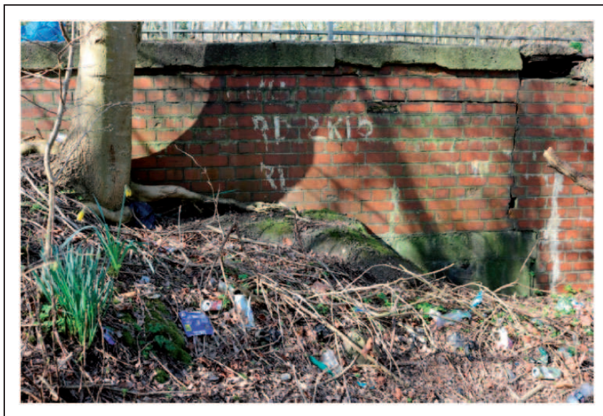
Figure 9. The brook passes under Barton Road Bridge and exits Kingsway Park to the west. Before culverting, this would have been a bridge over free-flowing water.
