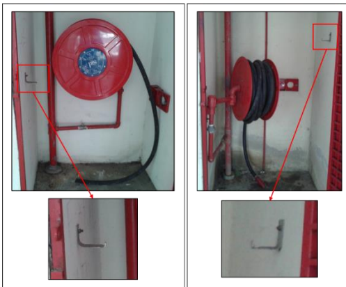
Figure 11: Missing portable fire extinguishers
